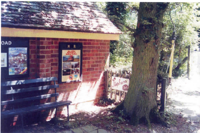
Haven Road Engine Shed, soon to be 30 years old, has been de-mossed and some tiles refitted.
