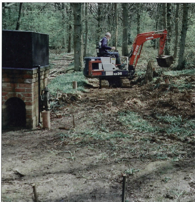
Work gets under way on our new loco shed at Haven Road
