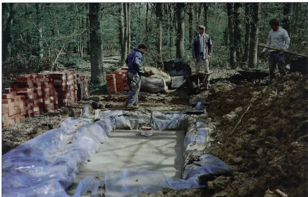
Construction is already well under way for the new loco shed at Bramble Hill
