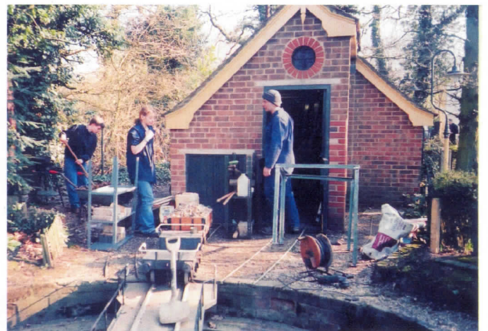
Workforce and Nick working on the support frame for Bramble Hill engine shed bench.
